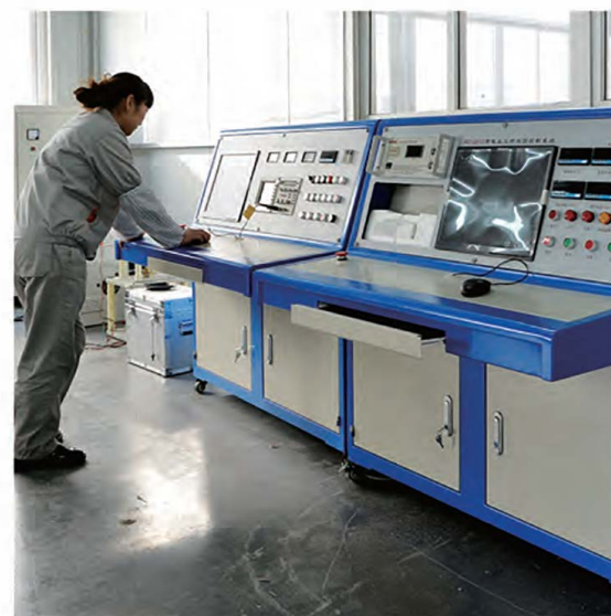
工频实验操作台 Operation table of power frequency test
